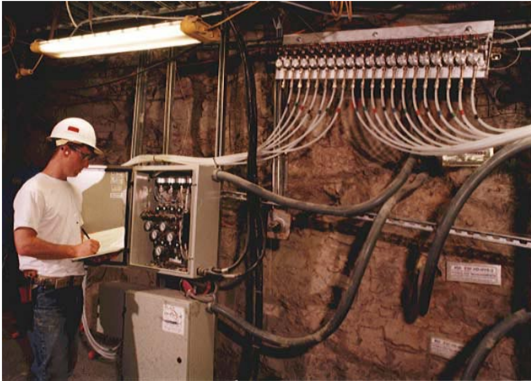
A technician inspects equipment used to inject a mixture of compressed air and a tracer gas (SF 6 , sulfur hexafluoride) into a borehole in the cross-drift. After some time, scientists will recover the gases from a separate borehole. By knowing the distance between the boreholes and the travel time for the gas, they can determine how fast fluids and gases move through the rock.
