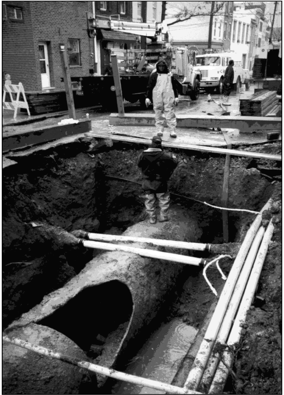
Figure 1: Decaying Drinking Water Pipeline in Philadelphia
