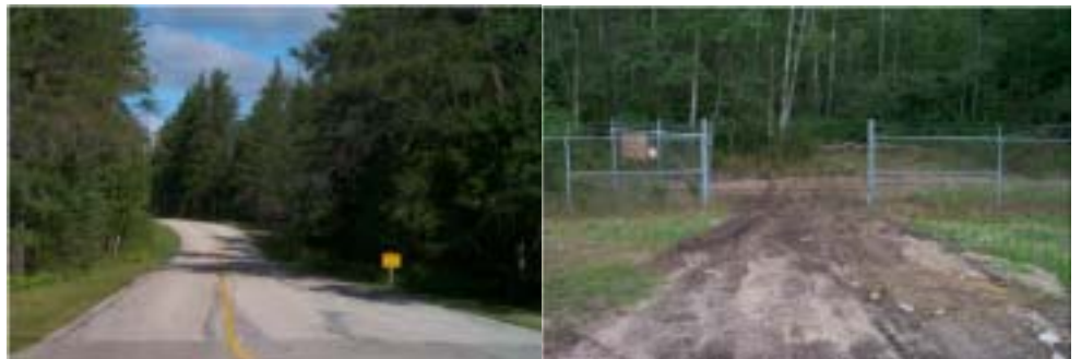
Roadways vary in condition from the good paved road at Seney NWR (MI) to the failed native surface road at Jordan NFH (MI)
