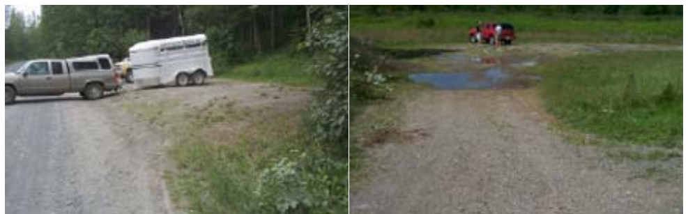
The parking lots at Kenai NWR (AK), on the left, and Erie NWR (PA), on the right, are examples of poor and failed parking lots that need to be improved.
